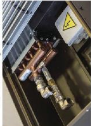
Heat exchanger "air-water"
