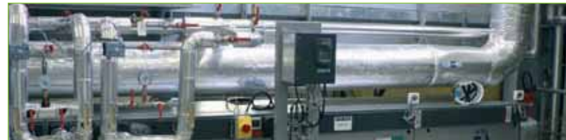
For \Delta T supervision on air handling system.
